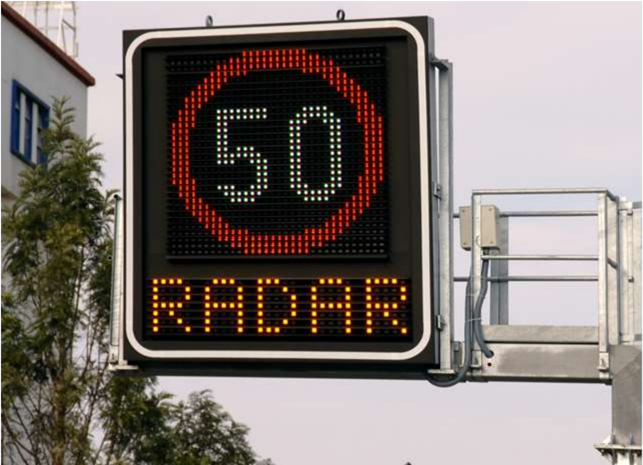
This smart road sign receives data and modifications to better inform drivers and prevent congestion or accidents.
